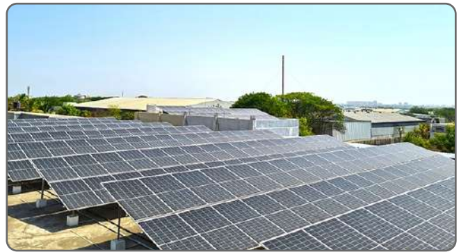
10+ MW | Industrial Rooftop
